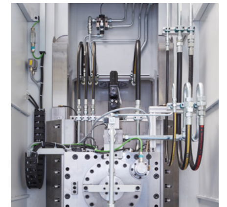
An important quality feature: Cleanliness and tidiness right through to final assembly
